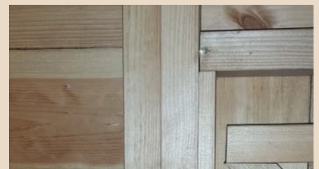
Door frame on both shiplap claddings have been doubled up to give extra strength.
