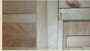
Door frame on both shiplap claddings have been doubled up to give extra strength.
